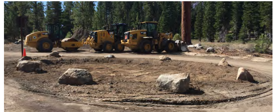
Figure 3–081—Permanent best management practices for water quality protection developed early in the construction process reduce the need for temporary strategies to handle runoff and pollution. This water-retention basin can be used both during construction and after.
