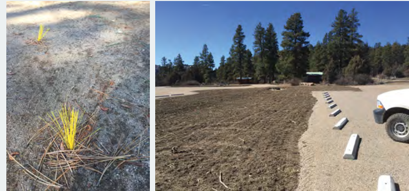
Figure 3-059—Delineate parking stalls by using finish grading stakes, “marking whiskers” (left), staked reflector domes, or wheel stops (right) to replace paint striping in aggregate or native surface parking areas. Staked materials require routine maintenance.
