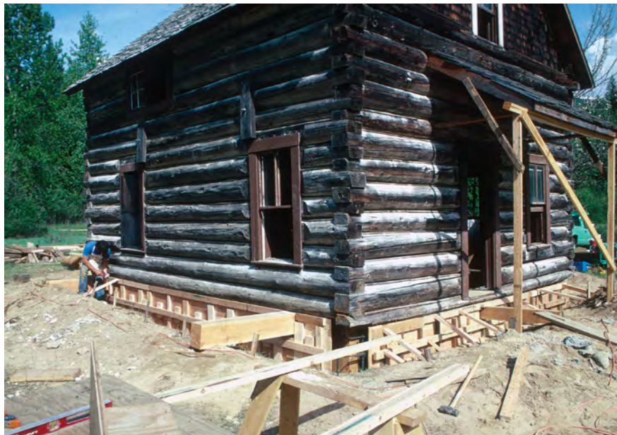
Figure 3–115—A group of workers employ traditional carpentry skills to restore a historic structure (top). New sill logs stabilize the base of a historic building (bottom).
