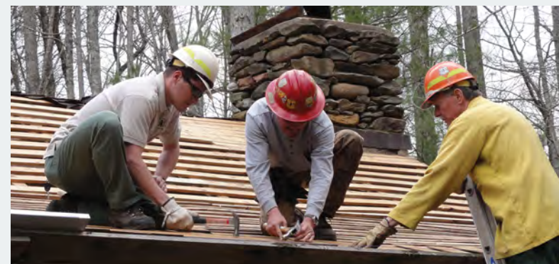
Figure 3-028—Preservation of historic structures includes work to protect and stabilize the property, such as replacing a wood shake roof.
