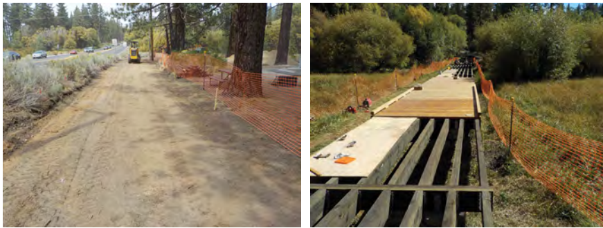
Figure 3–084—Fencing at the construction limits helps protect soils and other resources from unintended impacts from heavy equipment or other disturbances.
