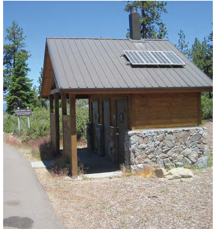
Figure 3–099—Photovoltaic panels and solar power reduce energy consumption and can provide power without installing electrical service.
