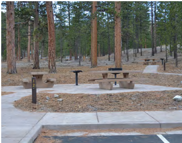
Figure 4-040—A reconstructed picnic site, before (top) and after (bottom). This project reduced the footprint of the site and decreased environmental impacts by clustering parking and individual picnic sites.
