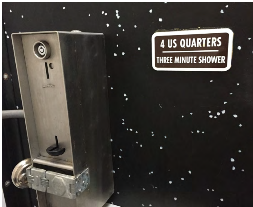
Figure 3–103—Consider using metered or token-timed shower facilities to limit water consumption.
