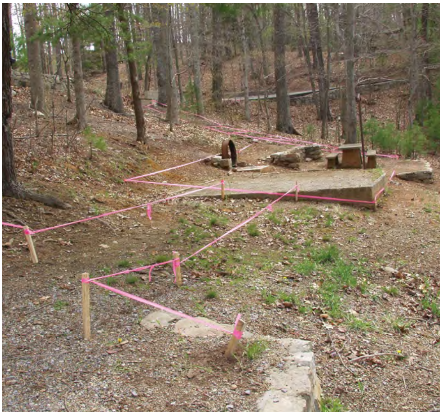
Figure 2–019—Staking out construction limits before breaking ground can often result in small improvements to a project.
