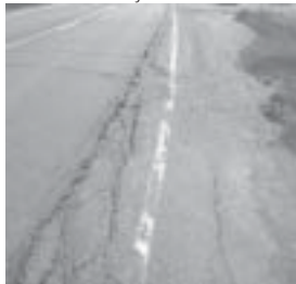
When resurfacing occurs over old concrete roadways, longitudinal cracks may appear where bicyclists normally ride.
