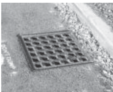
Parallel bar drain grates should be replaced with modern bicycle-safe and hydraulically efficient models such as the "vane" or "honeycomb" grates.
