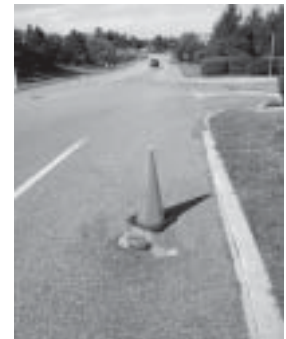
Remove uneven edges and grooves around utility covers and utility cuts.
