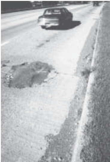
Small bumps and cracks that are barely noticeable to motor vehicles can cause a bicycle to crash or swerve.
