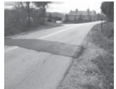
Backfill and compact utility cuts so that the cut will be flush with the existing surface.
