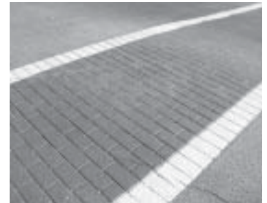
Textured crosswalks provide drivers with visual and audible clues that they are in a pedestrian environment.
