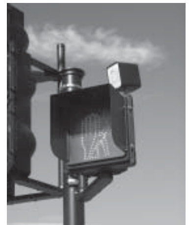
Auditory pedestrian signals may be provided when the need is established and an engineering analysis indicates the installation will add to the safety of pedestrians.
