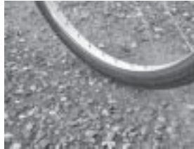
Aggregate too large for any use. Beebe Spur Rail Trail, Newport, Vermont (before replacement)
