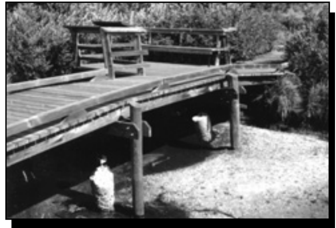
Figure 44—Know your soil conditions. Concrete end-bearing piles settled 1 to 2 feet here and had to be replaced with these log friction piles.
