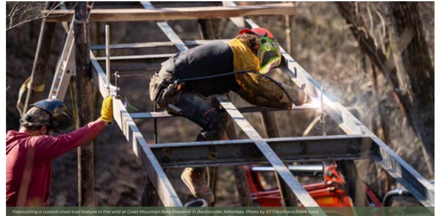
Fabricating a custom steel trail feature in the wild at Coler Mountain Bike Preserve in Bentonville, Arkansas. Photo by Eli Clesmann/Rock Solid
