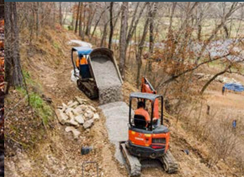
Chip-seal climb trail under construction at Coler Mountain Bike Preserve in Bentonville, Arkansas. Photo by Eli Glesmann/Rock Solid
