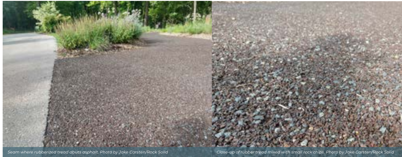
Seam where rubberized tread abuts asphalt. Photo by Jake Carsten/Rock Solid
