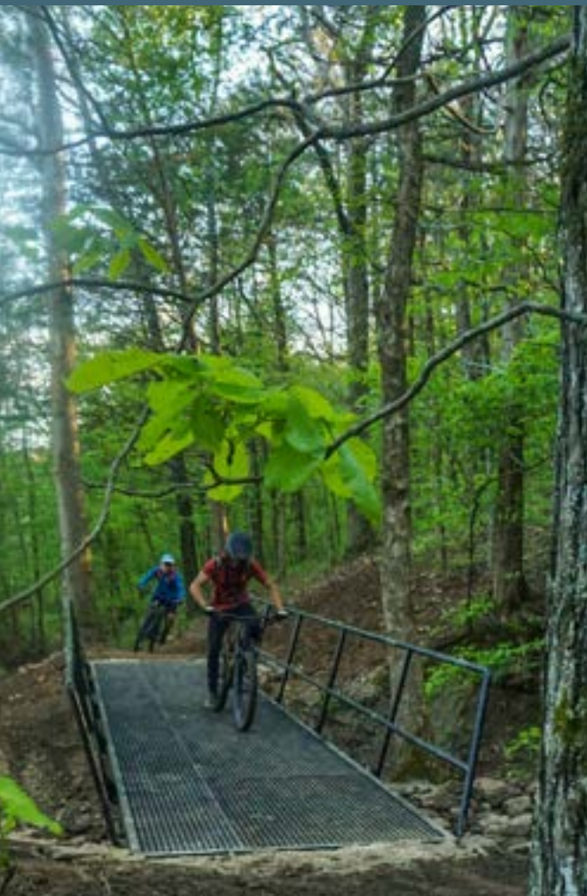
Prefabricated steel bridge at Devil's Den State Park in Winslow, Arkansas. Photo by Andy Flietstra/Rock Solid
