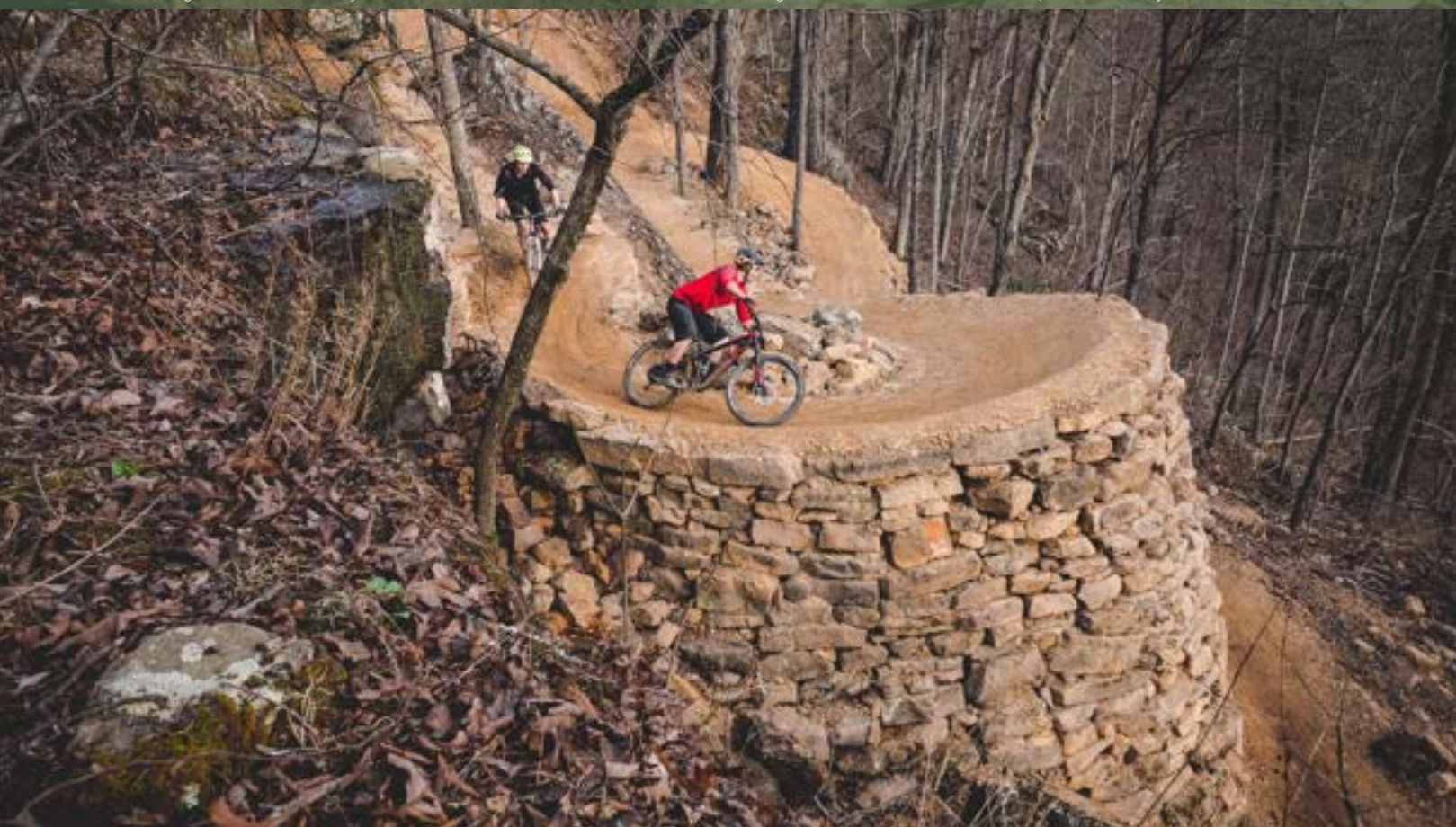
Construction of an extreme retaining wall was necessary to build the trail down a cliff wall. Photo by Hansi Johnson
