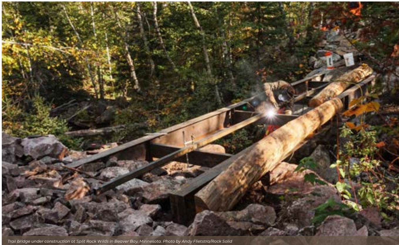
Trail bridge under construction at Split Rock Wilds in Beaver Bay, Minnesota. Photo by Andy Flietstra/Rock Solid
