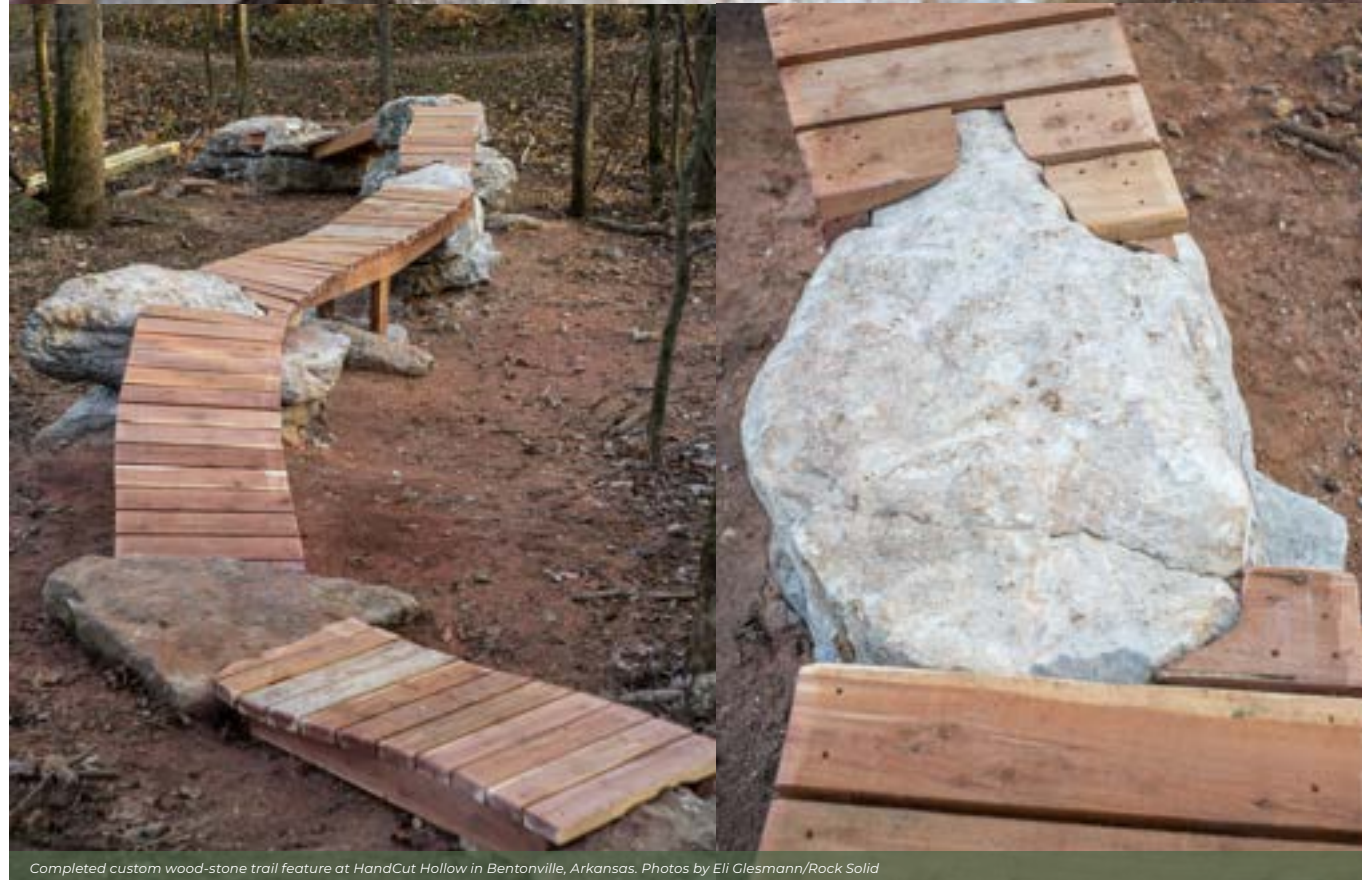
Completed custom wood-stone trail feature at HandCut Hollow in Bentonville, Arkansas. Photos by Eli Clesmann/Rock Solid
