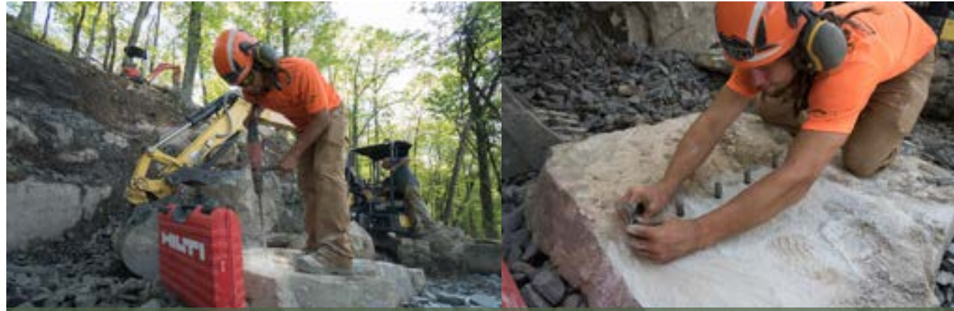
Rock drill prep for using feathers and wedges to split rock. Photos by Eli Glesmann/Rock Solid
