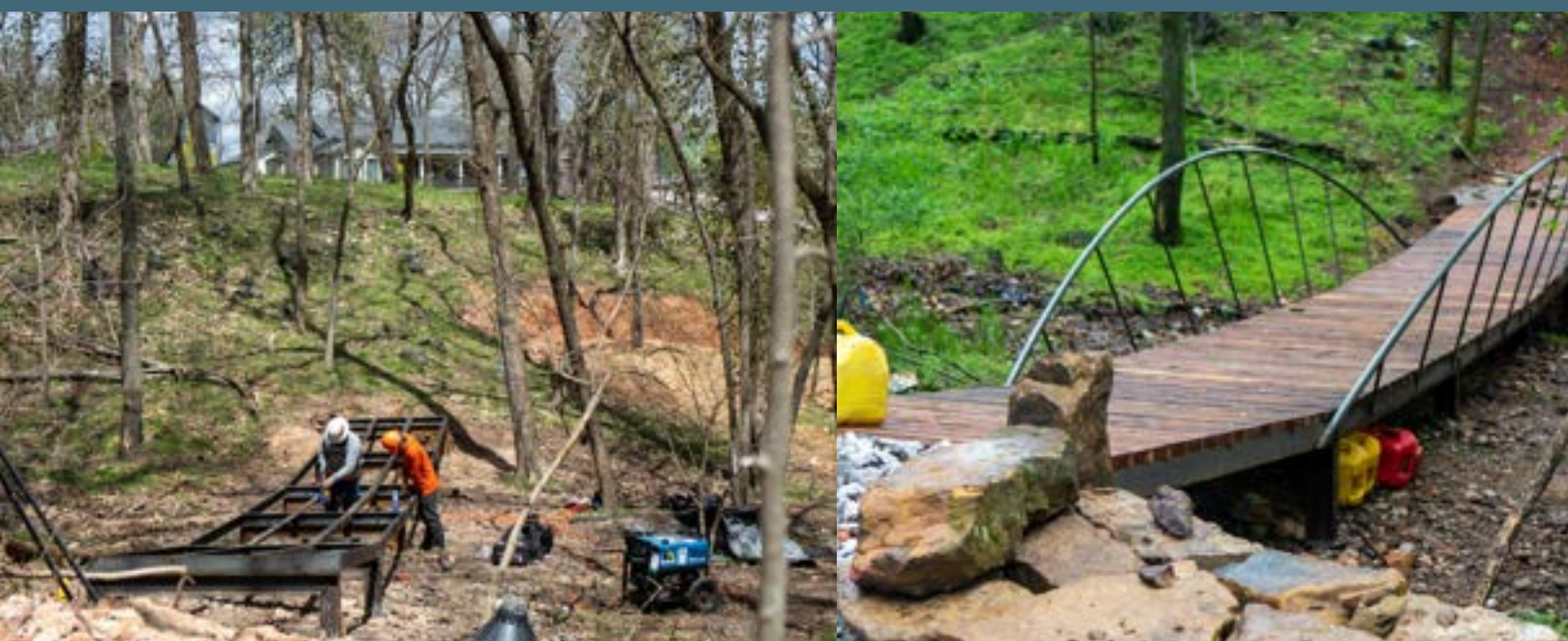
Steel-framed bridge with wooden decking at Headstart to Slaughter Pen in Bentonville, Arkansas. Photos by Eli Glesmann/Rock Solid
