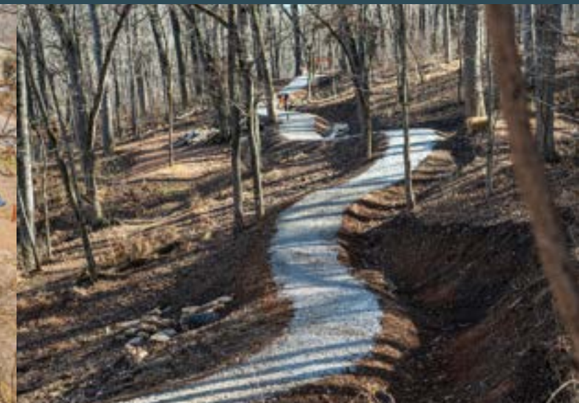
Chip-seal climb trail ready for top coats of liquid asphalt and fine aggregate at Coler Mountain Bike Preserve in Bentonville, Arkansas. Photo by Eli Glesmann/Rock Solid
