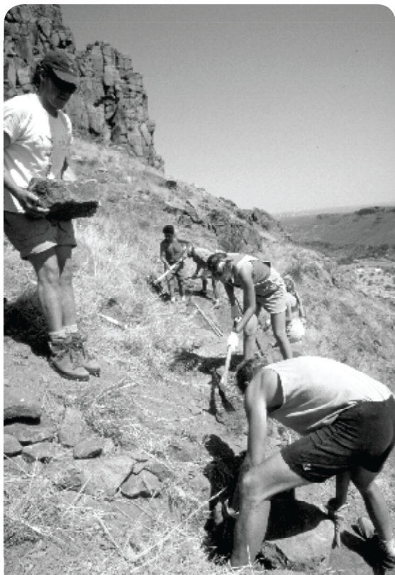
Volunteers on a trail-building project at North Table Mountain, Colorado. Funding for materials and trail design can also be obtained from climbing organizations. Photo: © Access Fund Collection
